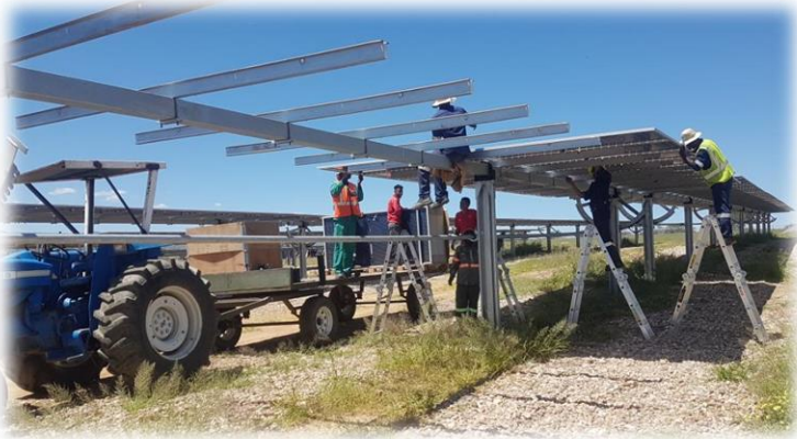
Namibia Poultry Industries Solar Farm completed 2022: Panel packing on modified trackers with reflective gravel underneath for bifacial effect of the panels increasing panel output by 5%.
