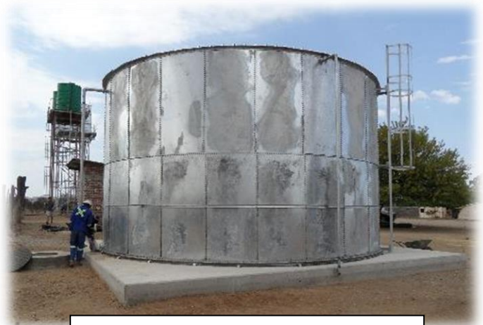
Circular ground mounted water Tank
