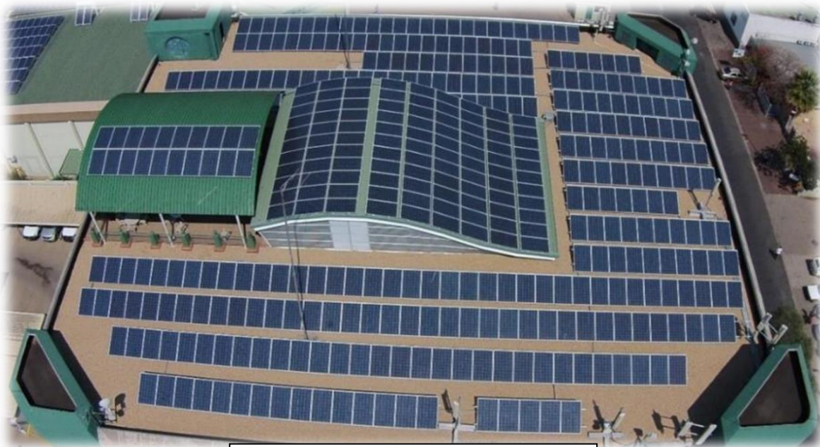
NamPower National Control Centre, Windhoek, Namibia: 103 kWp system
