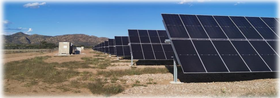
Finished Solar Park – 3 MW producing on average 23 000 kWh a day.
