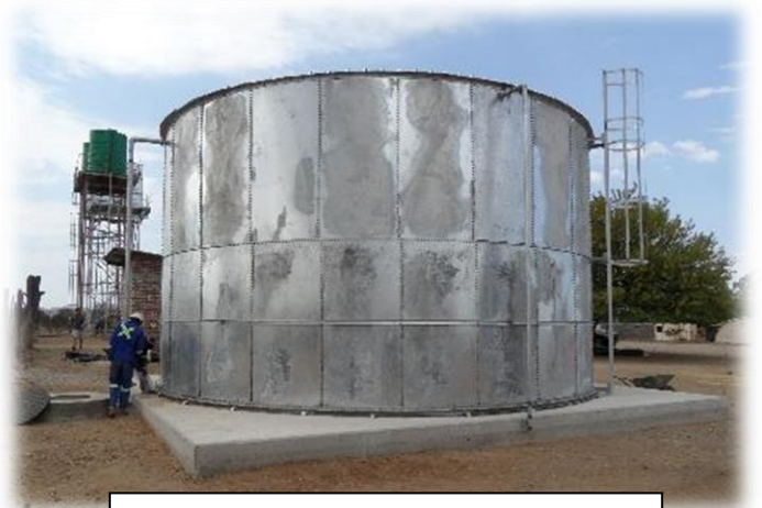
Circular ground mounted water Tank
